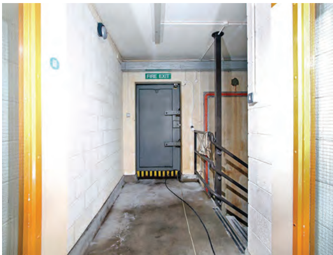
The emergency exit blast door and, to the right, stairs down to the lower level
